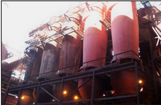
Severe abrasive wear typically repaired by welding in new wear plates every 4-5 months
